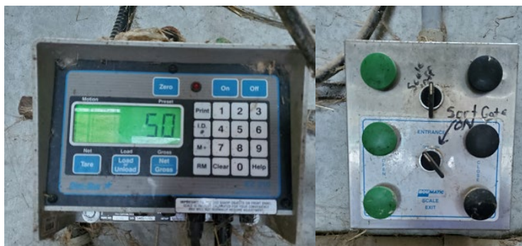
Fig 4&5. Control panels for platform scale, and gate control
